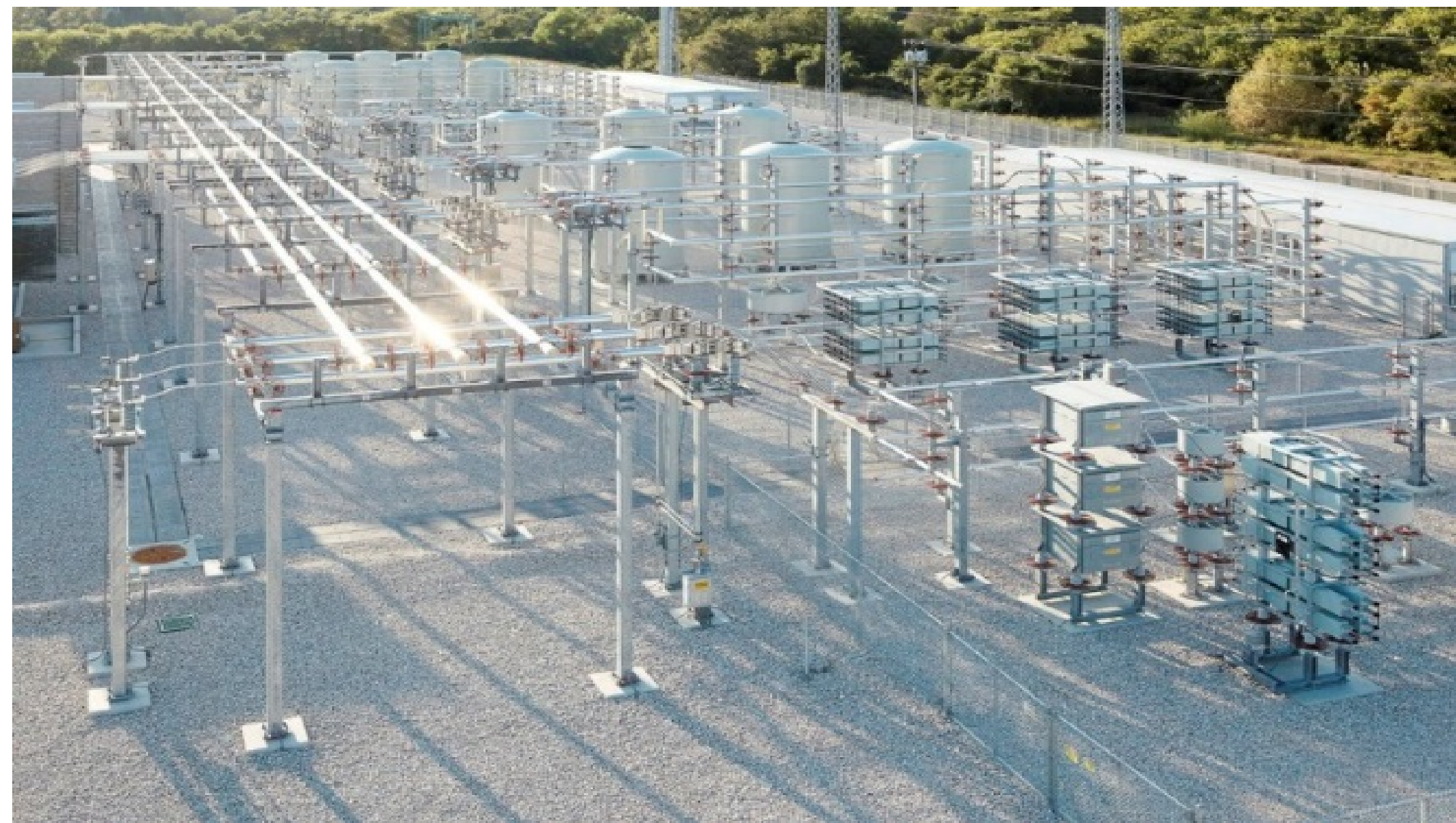
Figure 1. An ABB static var compensator outside Dallas, US. The three conductors to the left motivates the geometry considered (Fig. 3). Picture by ABB.
